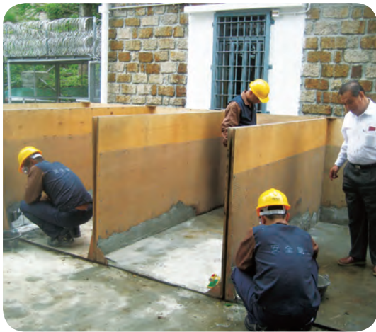
於裝修防水助理基礎證書課程，學員在導師指導下實習。 Trainees were practicing under guidance of trainer of Foundation Certificate in Decorative Waterproof Worker Training for Renovation.
